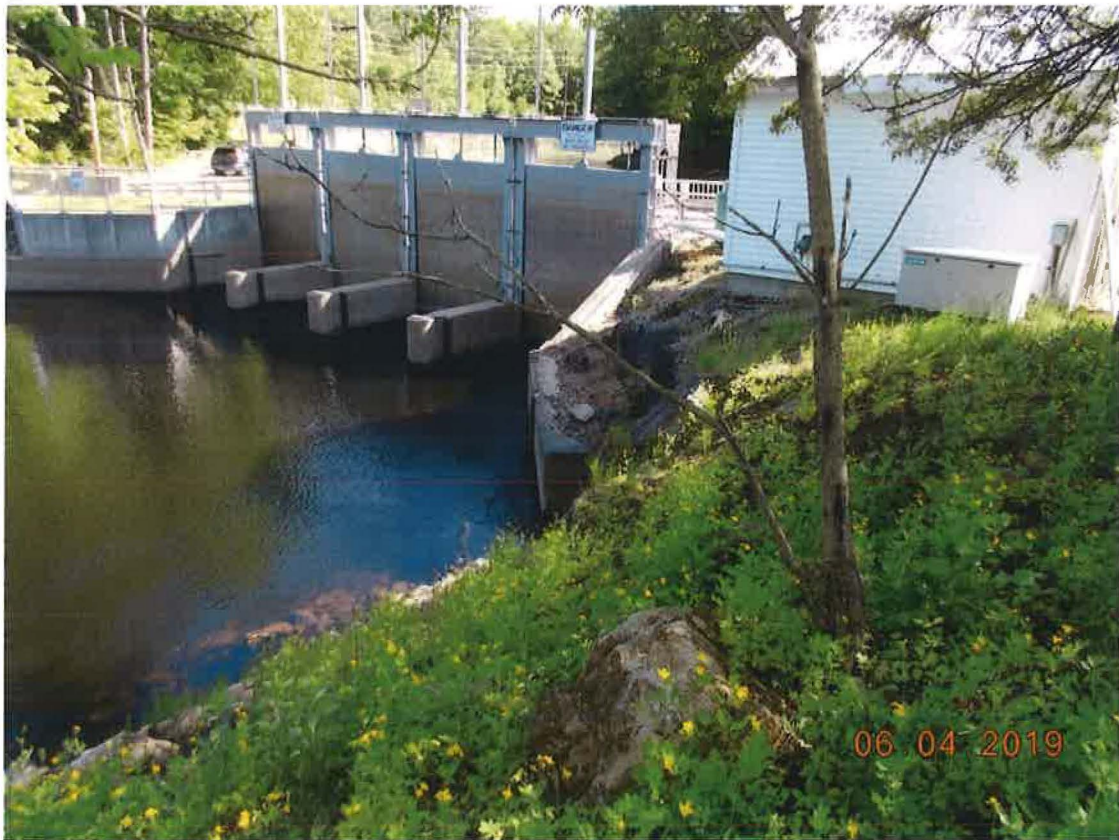
Figure 6. Rolfe Canal Gates
