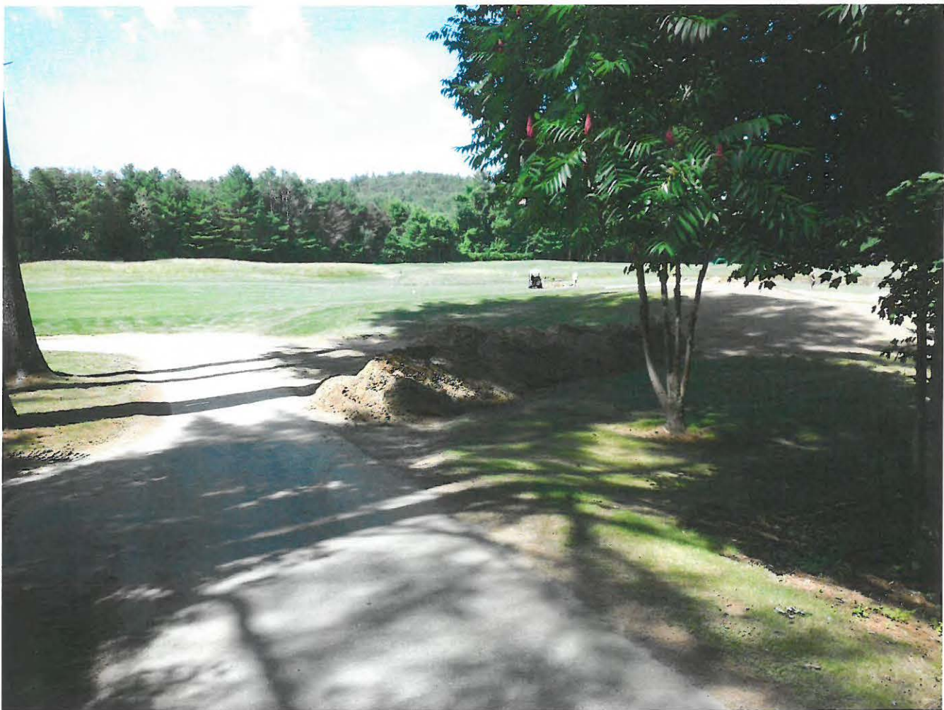
Observed at the time of violation, picture locate just over the tracks
